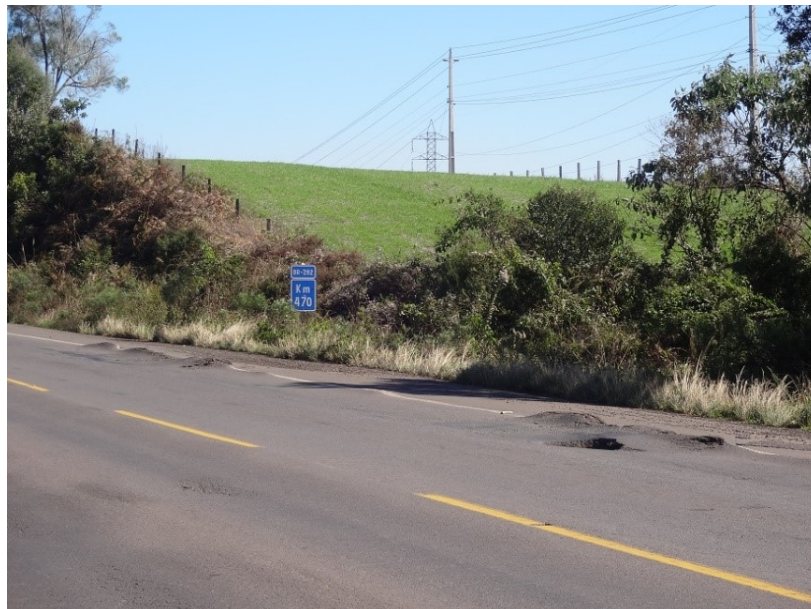
Figura 14: Buracos e recalques Rodovia BR-282/SC, no km 470
