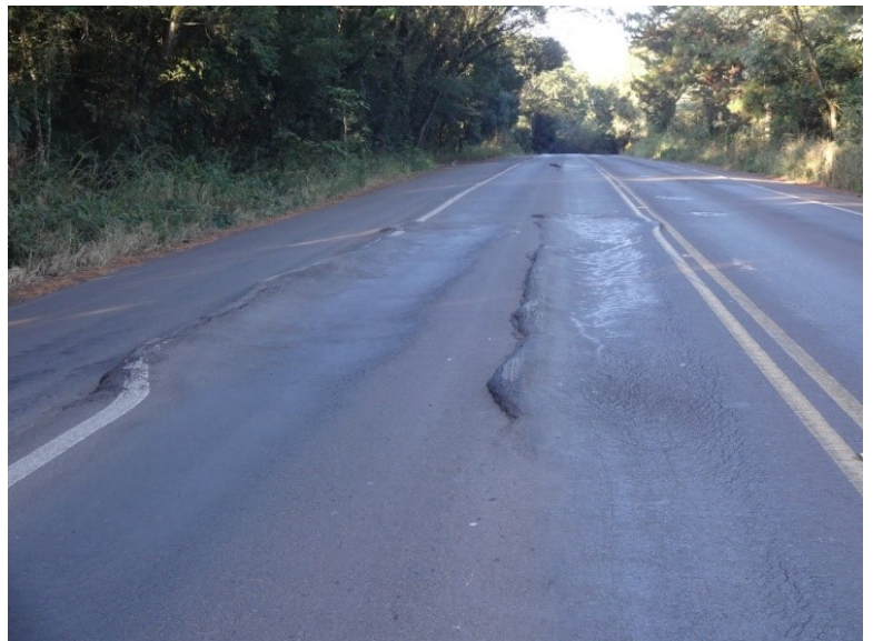
Figura 39: BR-282/SC km 593,0 – Afundamentos e recalques
